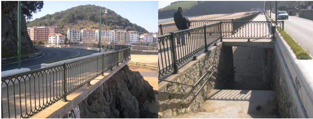
Fig.IV-14 and IV-15. (Left) Side platform on the rocks (Right) Stairs down to the beach (Photo by I. Español).
