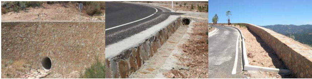
Fig. 60, 61 and 62. Sandstone is a consistent material which being used in different road elements (retaining wall, drains and parapets) builds up a sense of identity (Photos by I. Español).
