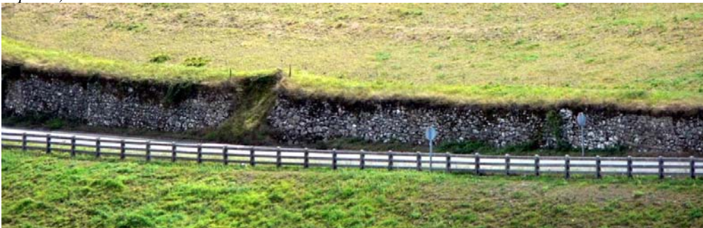
Fig. 25. A traditional stone wall works as a retaining wall for the road cutting, while the embankment has been successfully naturalised by grass. (Photos by I. Español)
