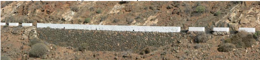
Fig. 26. The road platform is held by a retaining wall concealed under a finishing of traditional stone walling. Traditional stone walling and an old-fashioned white parapet provide a positive result in functional and landscape terms. (Photos by I. Español)
