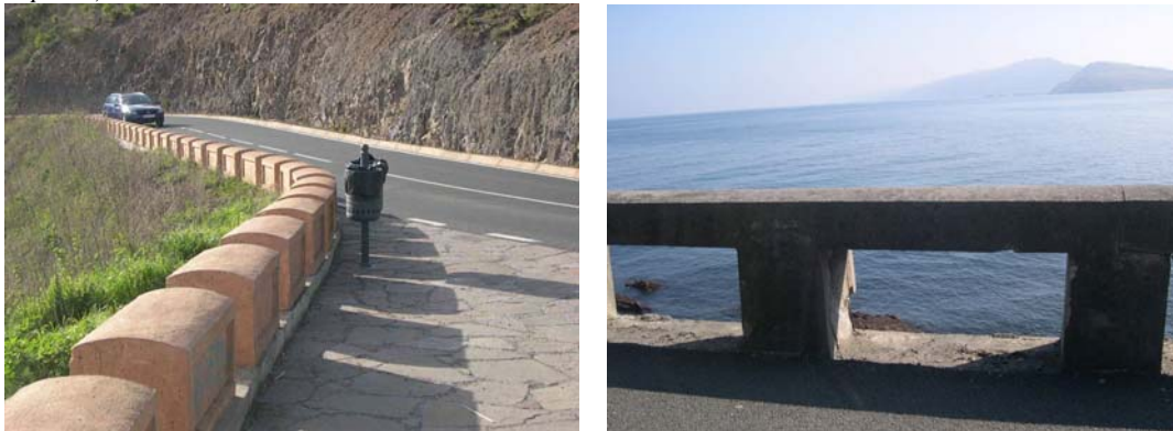
Fig. 20 and 21. Traditional parapets newly built in the old-fashioned way (left,) or preserved in their original state (right,) provide a familiar look (Photos by I. Español).
