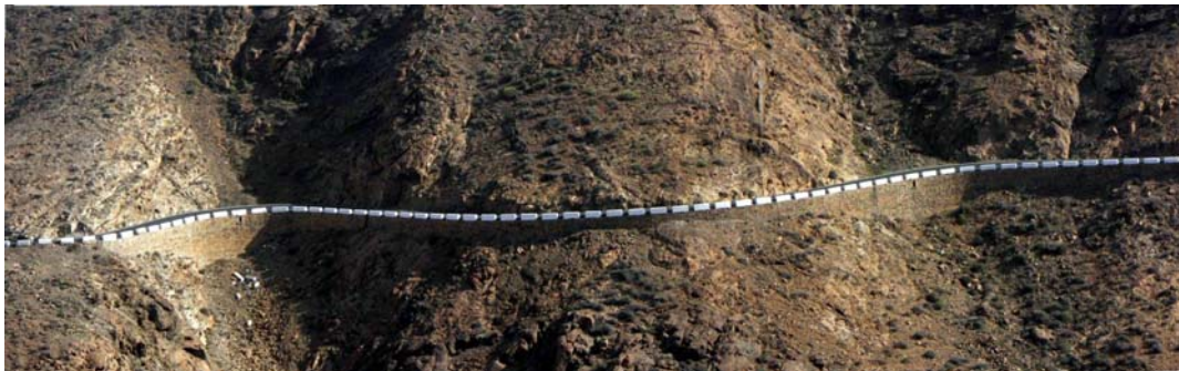
Fig. 80. Traditional character elements, such as a teeth- like safety barrier and retaining walls made from local stone, encourage a positive landscape integration. (Photo by I. Español).
