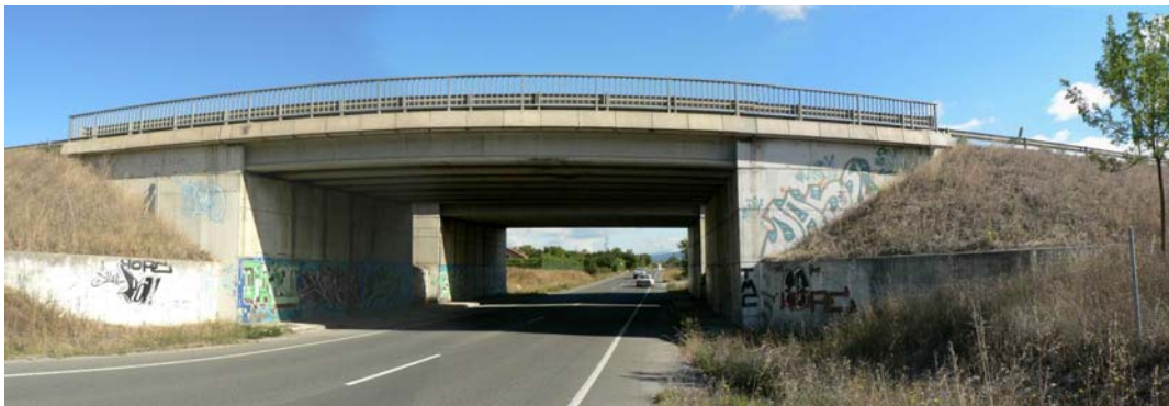
Fig. III-2. A conventional bridge allows the A-3002 to cross the A-1 ring road motorway. (Photo by I. Español) Note urban graffiti on the walls.
