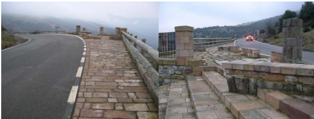
Fig. 52 and 53. Scenic viewpoint. (Left) Parking lane and access. (Right) Parapets and barriers for pedestrian safety. (Photo by I. Español).
