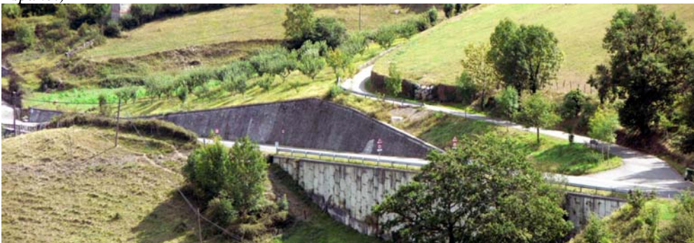
Fig. 24. The picture above shows a road whose embankment is supported by a prefabricated slabbed wall partially hidden behind a tree on the right side of the picture. The road cutting on the same stretch leans on an inclined concrete retaining wall which helps to support both the slope and a ramp. (Photos by I. Español)
