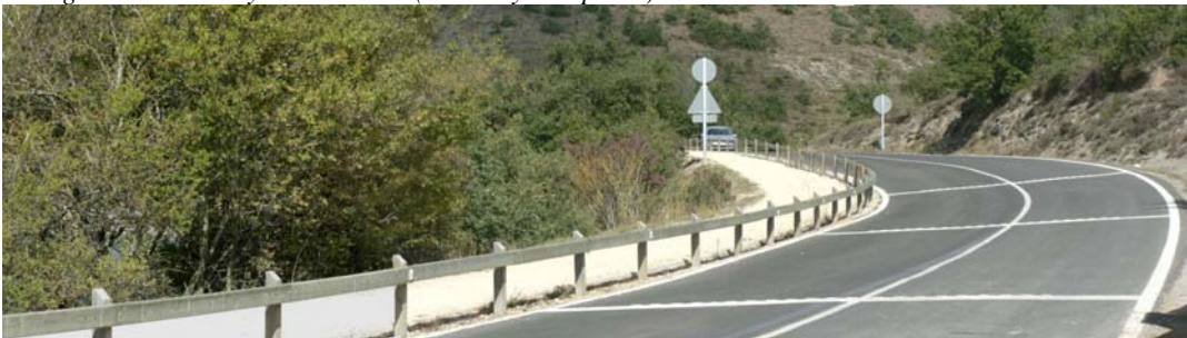
Fig. III-11. Speed reduction marks on the road and a low safety barrier create more footpath safety and comfort. (Photo by I. Español)
