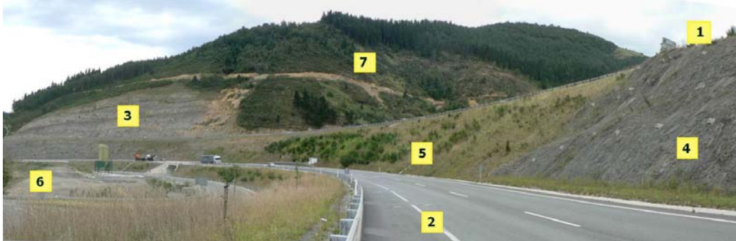
Fig. 76. Construction of a separated dual carriageway to expand capacity. (Photo by I. Español) Earthworks, particularly those of high-speed and high-capacity roads, determine road presence in
