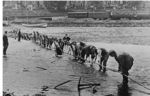
The laying of a cable in the River Esk © Sutcliffe Gallery ( www.sutcliffe-gallery.co.uk )
